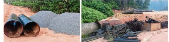
A check by StarMetro found two piles of gravel and steel culverts at the site. (Right) Earthworks at the site in Bukit Enggang have been going on since August last year.
