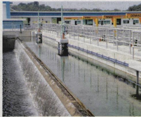
Part of the Langat 2 LRA, namely Stream B, had been operating since Dec 21, 2019, but only at a capacity of 430 MLD
