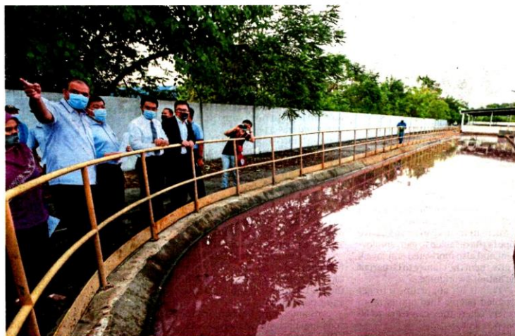
State Tourism, Environment, Green Technology and Orang Asli Affairs Committee chairman Hee Loy Sian (third from left) at the Indah Water Konsortium sewerage plant in Rawang yesterday. PIC BY ASWADI ALIAS
