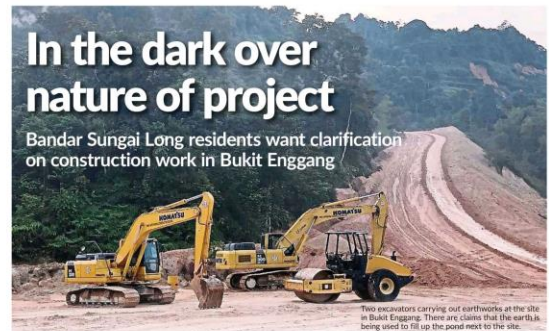
Two excavators carrying out earthworks at the site in Bukit Enggang. There are claims that the earth is being used to fill up the pond next to the site.
